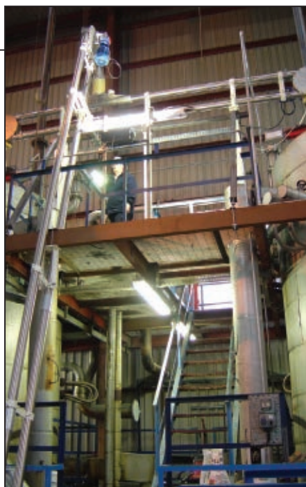
FIGURE 2. This aero-mechanical conveyor (AMC) operates high up into the roof area. In this situation, rope tension maintenance could be more difficult without the use of scaffolding or a mobile access platform
